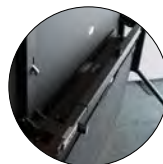
Kabelkanal cable duct
