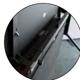
Kabelkanal cable duct
